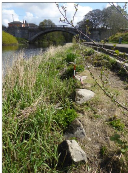
Plate 2 View of Lucan bridge in the background and the possible revetment (CH1)
