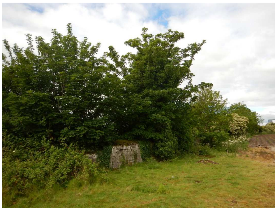
Photo 2. Semi-mature and early mature Sycamore trees growing out of or very close to the old masonry wall along the northern perimeter of the site.
