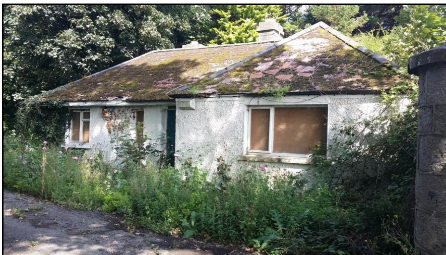
Plate 2. Potential bat roost location: Abandoned gate lodge on northern side of the R403.
