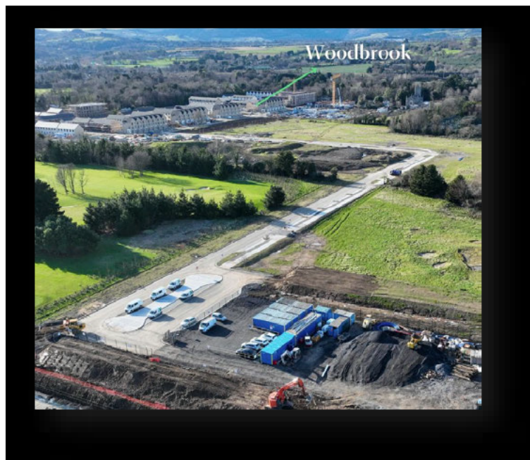
Image above: Aerial Photograph of the Woodbrook Dart Station while under construction with the serviced housing developments, for which it was built, in the background. (Source: Google Images.)
