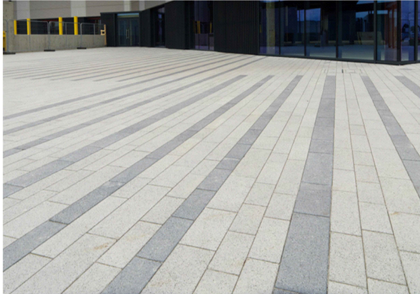
Primary footways: Pcc granite aggregate paving blocks
