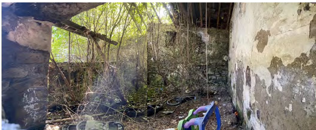
Plate 15: Top from left: General view of Outbuilding C7 - East elevation, west elevation showing existing openings. Centre from left: Existing door arrangements and internal view looking north. Bottom: View of south section of C7 showing internal arrangement and roof
