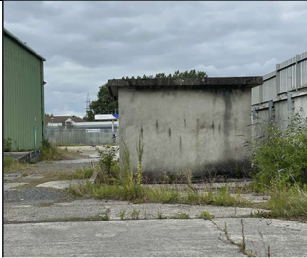
Existing ESB Substation to be relocated.
