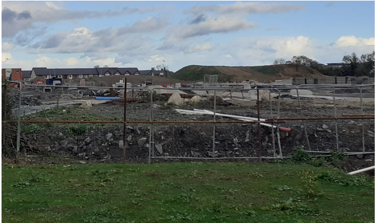
Figure 3-2: The construction area of the site, as seen from the western boundary.
